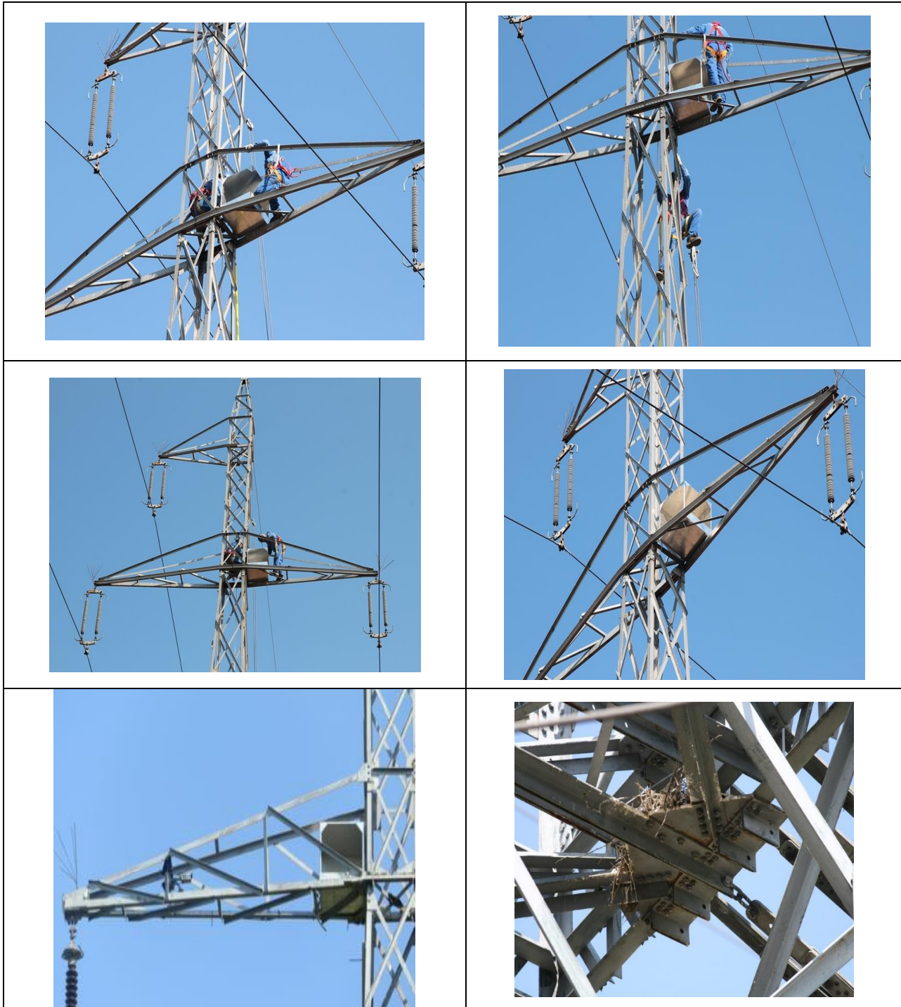
Figure no.33. Images 20 of the installation of nests on pillars of the OHL.
