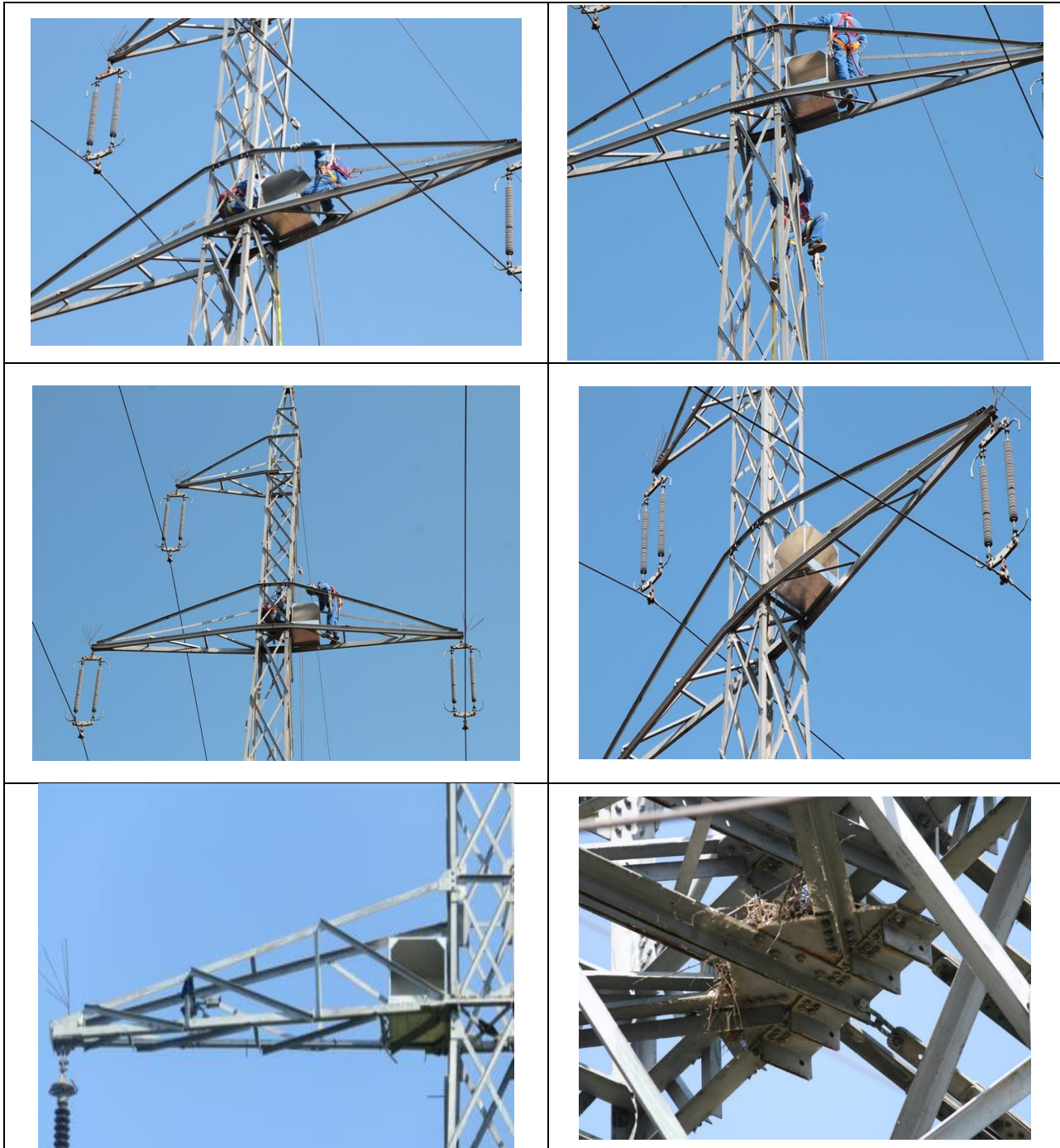
Figure no.33. Images 31 of the installation of nests on pillars of the OHL.
