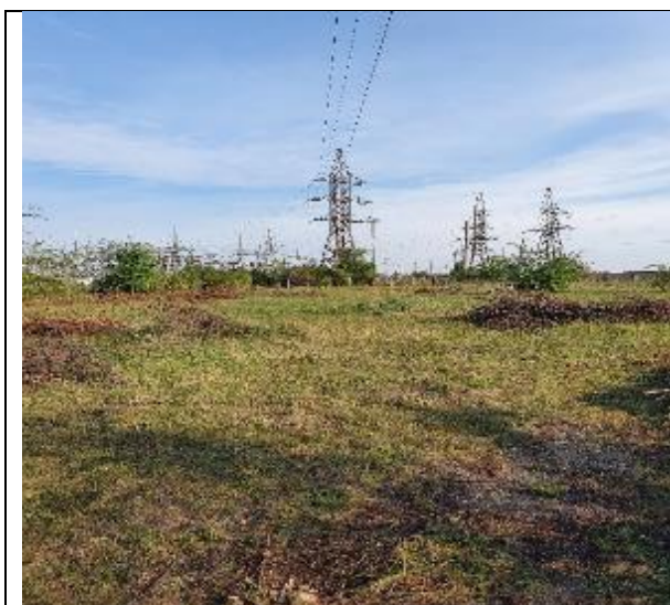
Fig. 3-7: Removed bushes under the 35 kV inside of the Chisinau SS
