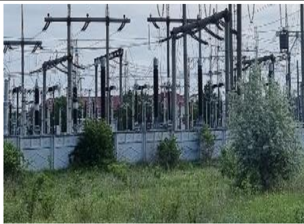
Fig. 3-9: The view of the Chisinau SS and with fence around
